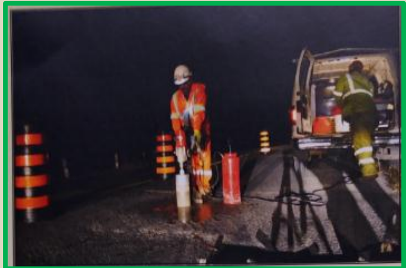
Sampling and onsite testing of badly damaged roadway or emergency remedial compaction
